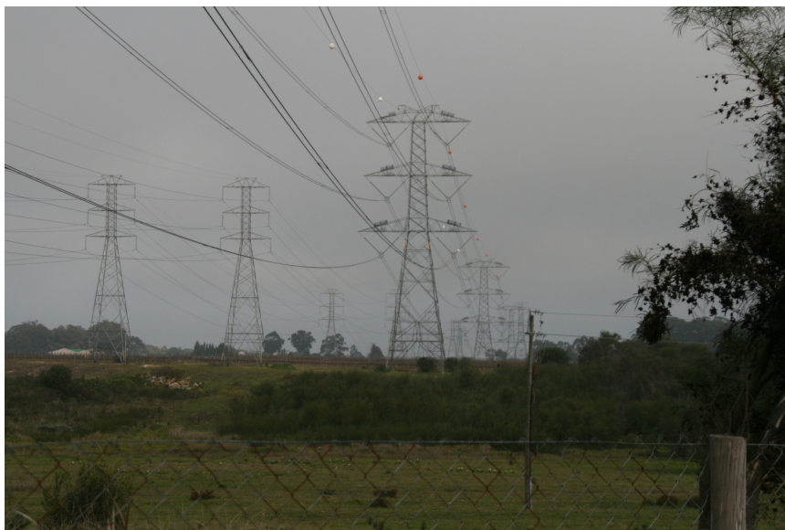
Figure 3.3: Photograph of conductors strung between transmission towers.
