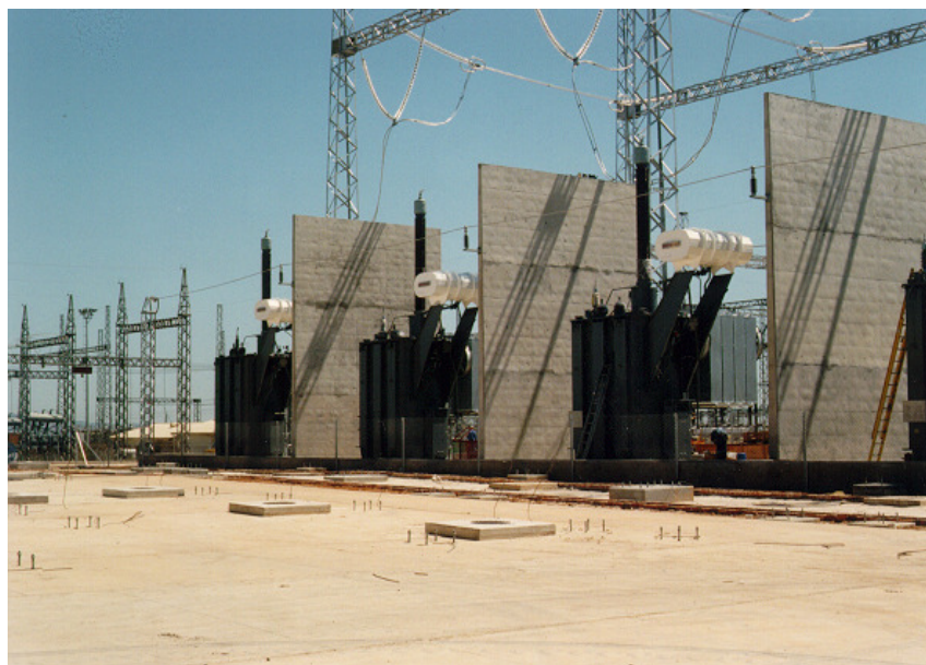
Figure 3.5: Transformers at a Substation.
