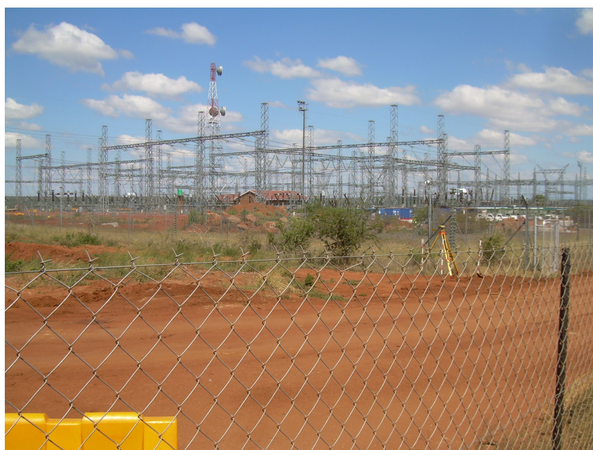
Figure 3.4: Photograph of a Substation, which transforms electricity from high to low voltage for consumer use.
